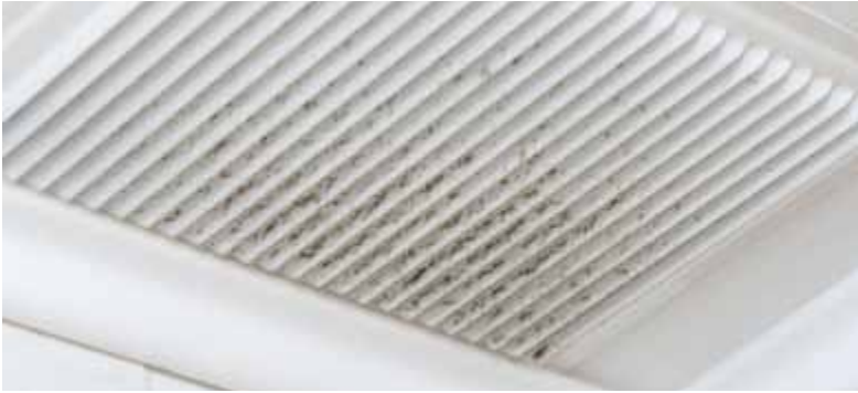
Air conditioning system. © Shutterstock
